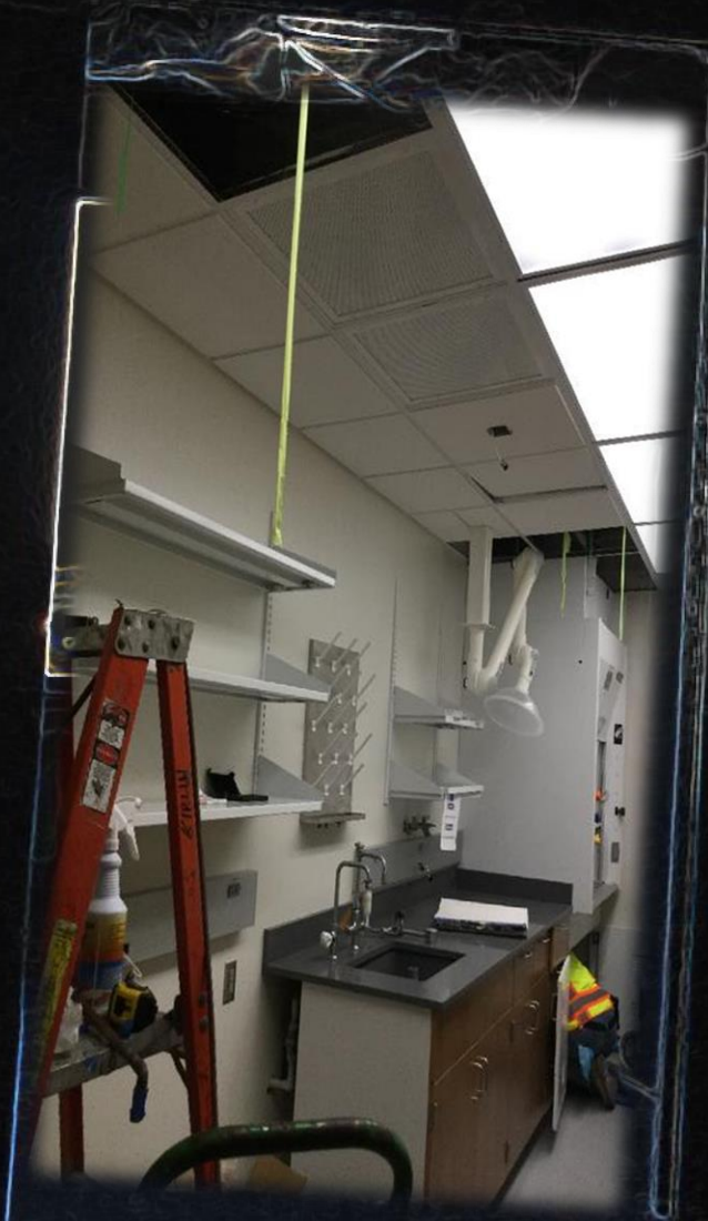
Subcontractors are installing lab casework. Metal shelving, sinks, lab connections, etc. are being set.
