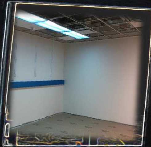
Labs and research rooms are well under way. Electrical raceways are being installed.
